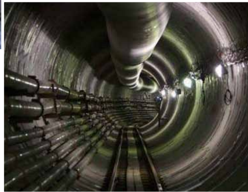
12" (300mm) & 14" (350mm) R-88 couplings used in tunnel boring / mining application. The pipe line delivered a bentonite water mixture while the outflow was an aggressive rock and mud slurry, Portland, Oregon, USA
