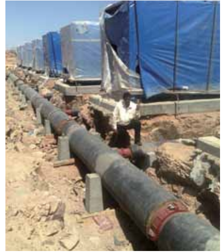
36" (900mm) Model R-88 couplings used in an HVAC chilled water line for a major university, Saudi Arabia
