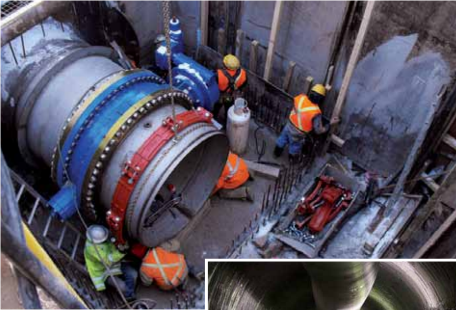
72" (1800mm) Model R-88 couplings used in a domestic water treatment plant, Ontario, Canada
